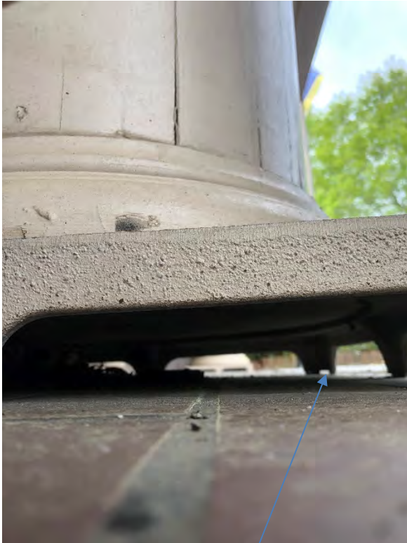
FRICION BASE PLATE. NOT ACCEPTABLE PER BUILDING CODE
